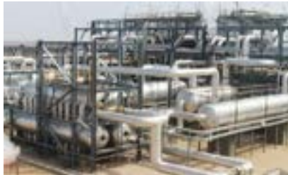
50MWe steam generation system
